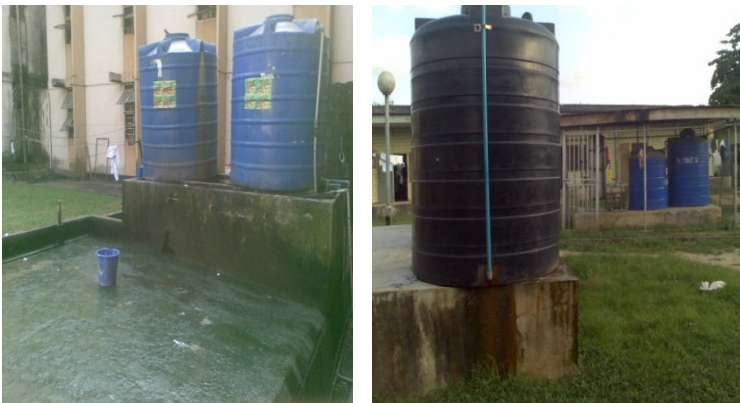
Plate 2: Showing the provision of water tanks as condition of facilities a storage medium
