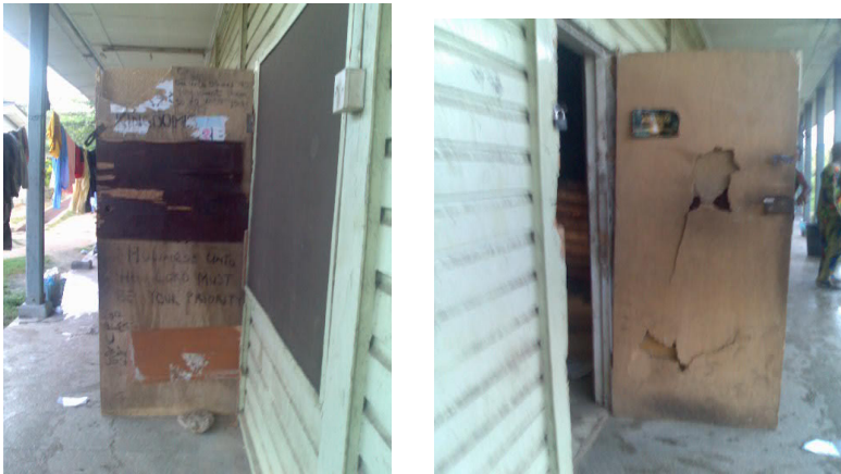
Plate 1: Showing the poor condition of doors in the students hostel (El Kanemi Hall).
